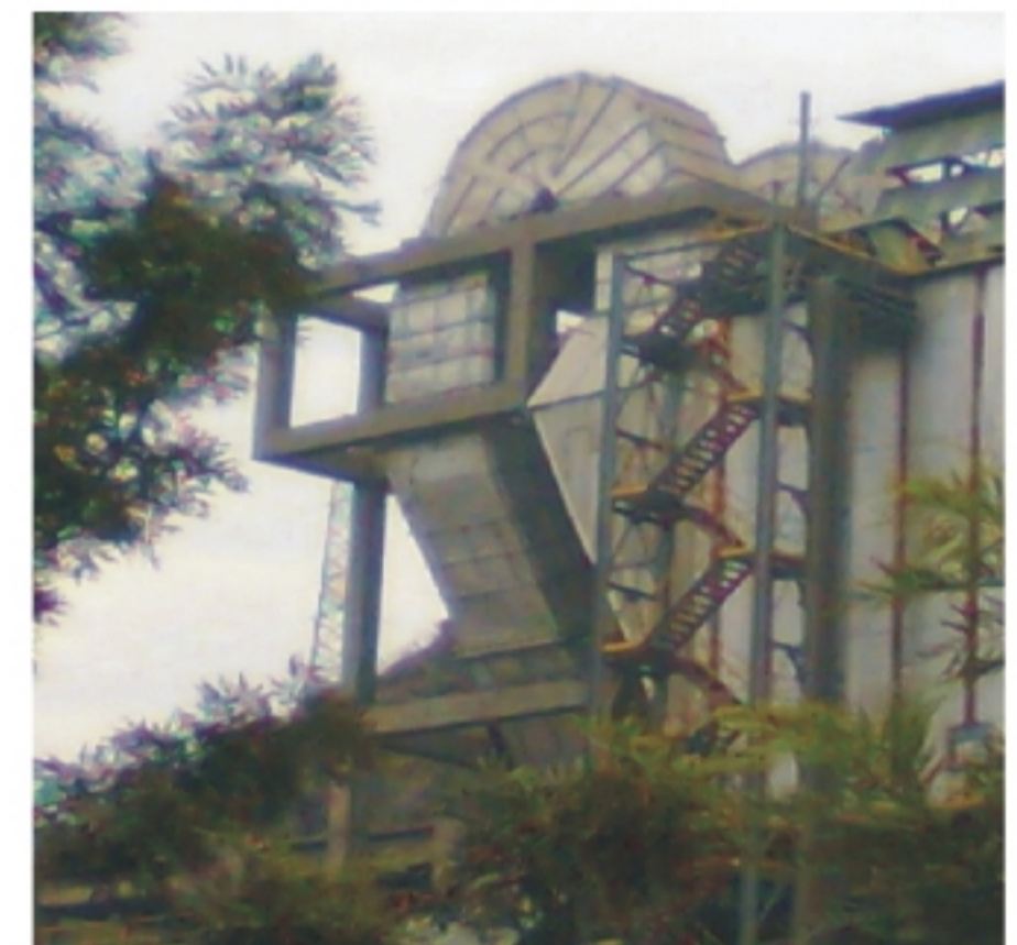
Cooler Duct For Cement Plant
